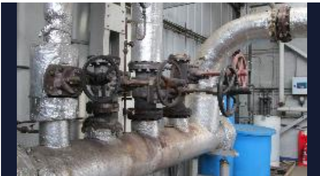
Visible-light view / Exposed steam valves
